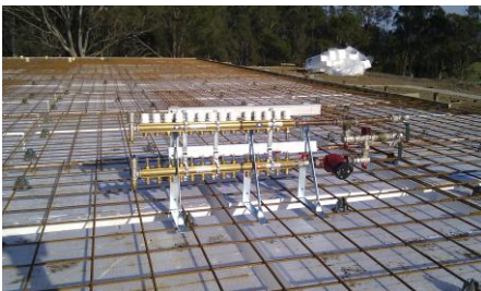
IN SLAB MANIFOLD
