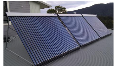
SOLAR EVACUATED TUBES
